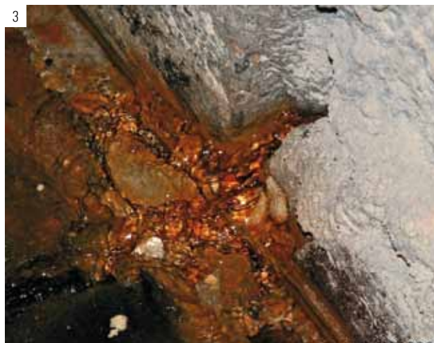
1 Cavity behind ceramic wall lining 2 Dismantling to the old tunnel's bare concrete 3 Leakages in the block joints
