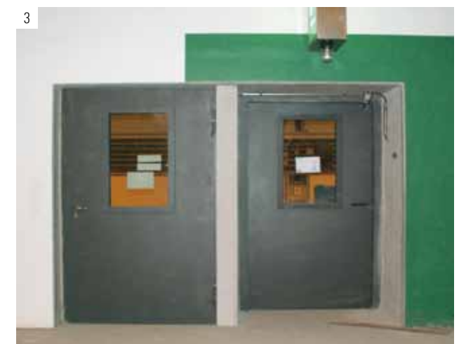
1 Old operation and traffic technical installations, emergency doors 2 Widening of emergency doors 3 New emergency doors in the middle wall between tunnel shafts
