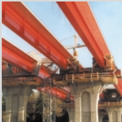
Oberhartmansreuth viaduct, installation of VFT girders, bridge deck constructed later with formwork carriages
